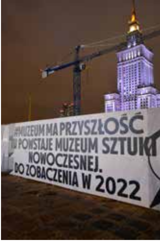
Fig. 3: Construction site of the Museum of Modern Art in Warsaw in 2019. Text on the fence says: #museum has future. The Museum of Modern Art is constructed here. See you in 2022. Photo: K. Jagodzińska.
