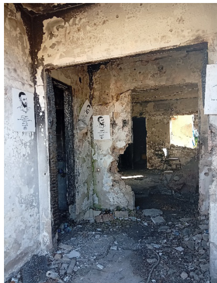
Fig. 1: Destroyed House in Kibbutz Kfar Azza. Photograph: Dalya Markovich.
