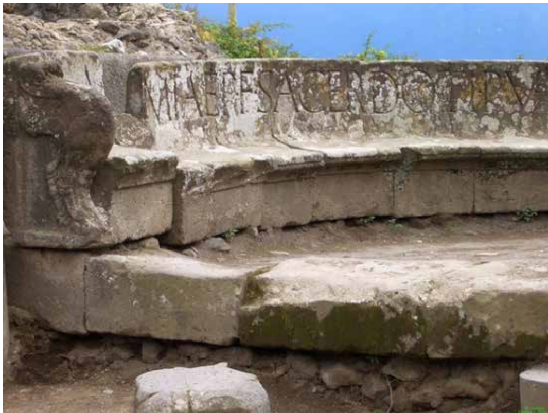
Fig. 5: Detail of the damage to the Schola of Mamia, Pompeii. CC: Jörn Kobes.
